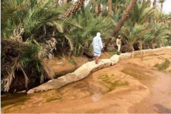
Timia Cooperative's protective dike, financed by USADF and recently built around the date palmeriaes
